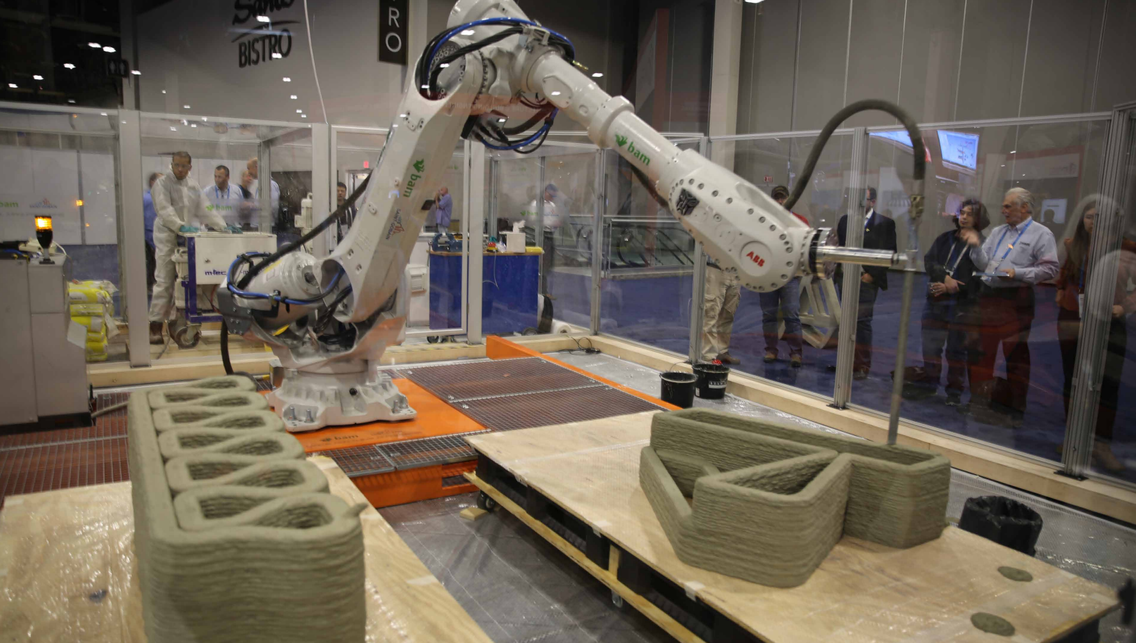
Courtesy of Autodesk: Royal BAM Group's BAM Infra and Saint-Gobain Weber Beamix demonstrate the use of a 3-D printing robot for offsite manufacturing for construction.
