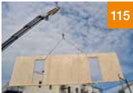
Transformation through a production system
